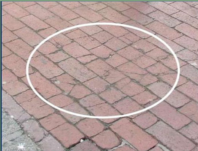
Attribute = Block Footpath Defects
